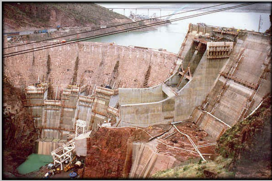
Arizona's Roosevelt Dam in 1994, under renovation. You can see the stone blocks within.
